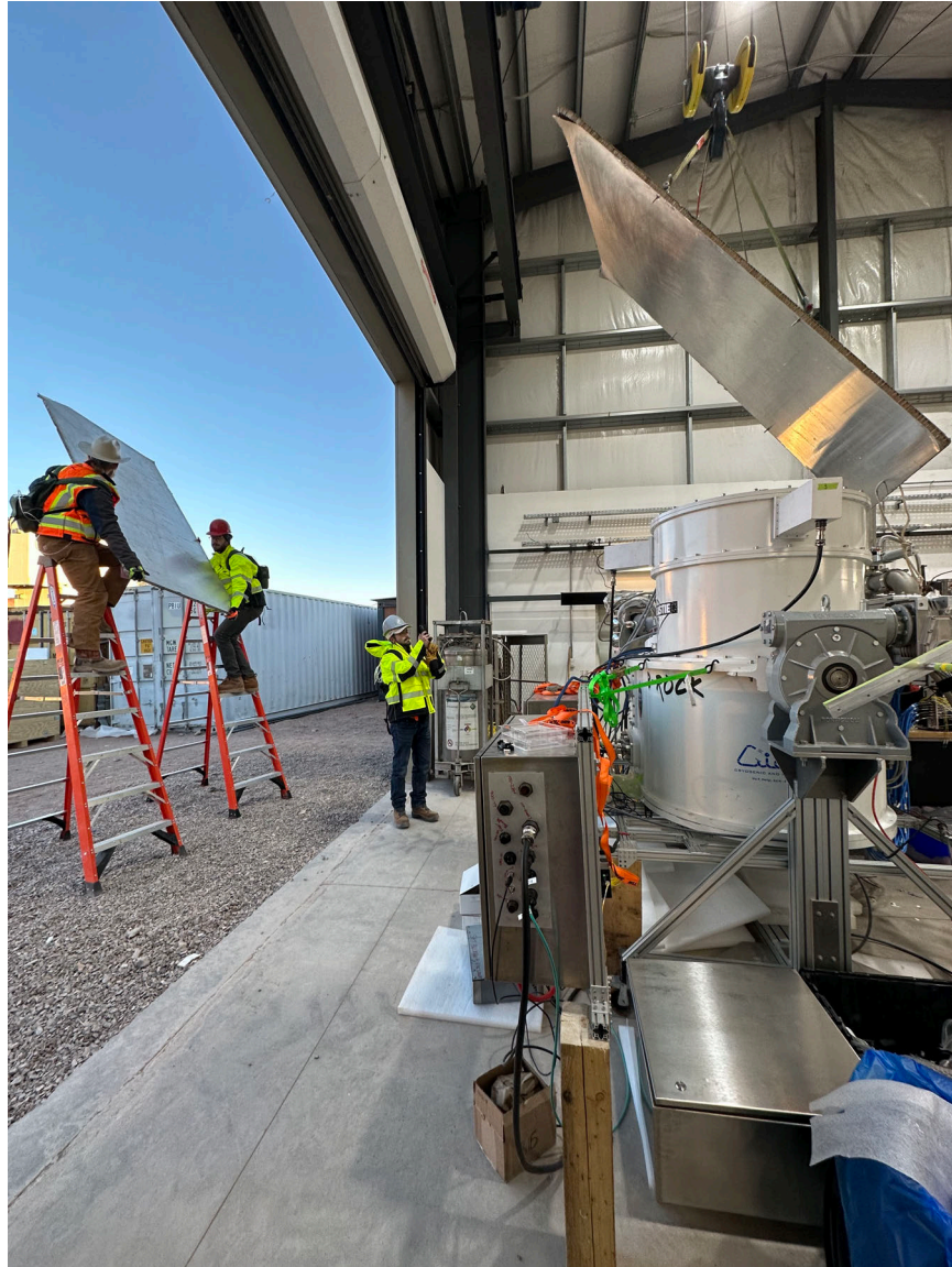
Figure 52. Two mirrors are used to attempt to direct sky light onto the SAT-MF1 focal plane during the site highbay cooldown.
