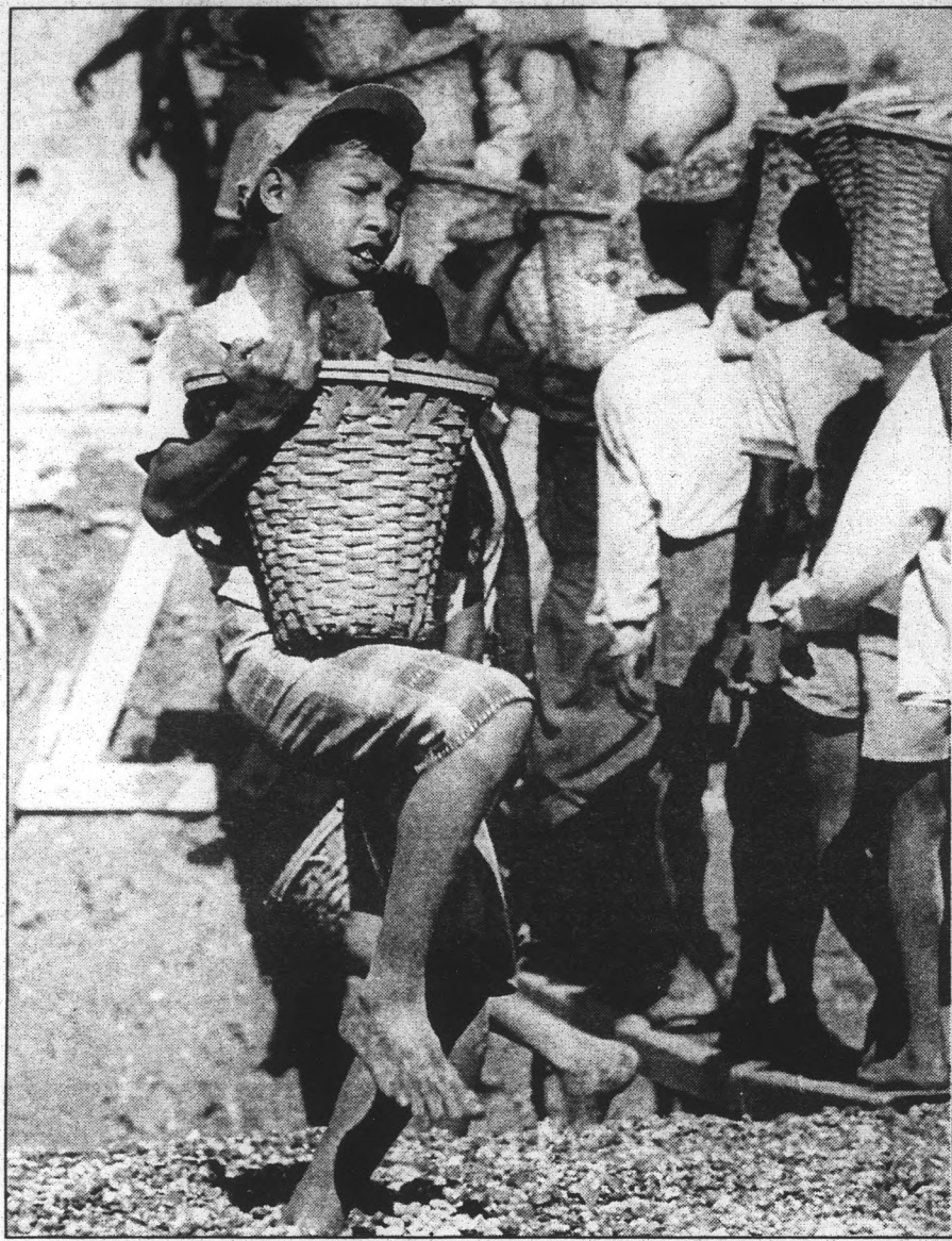
Thaksina Khaiakew/Associated Press A Burmese boy hoists a basket of sand onto his shoulder at one of the construction sites in downtown Rangoon, the Burmese capital, Sunday. Burmese children as young as five are commonly seen here as workers helping the parents fending for their family. They each earn at least 200 kyats ($1) a day. Burma was granted membership of the ASEAN last year.
