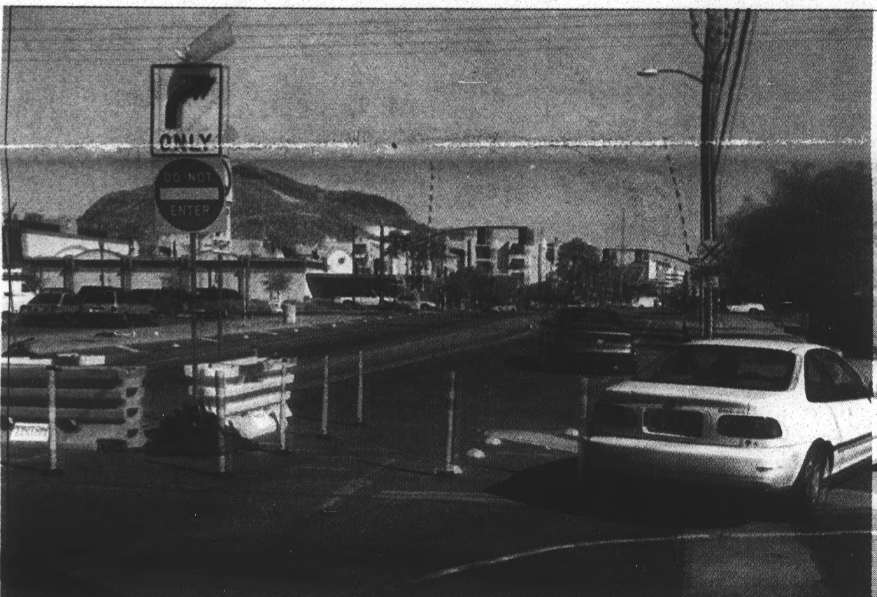
Barricades at the intersection of Fifth and Farmer have proven to be a nuisance to Tempe Drivers. Despite the detour, drivers continue to proceed around the barricade.
