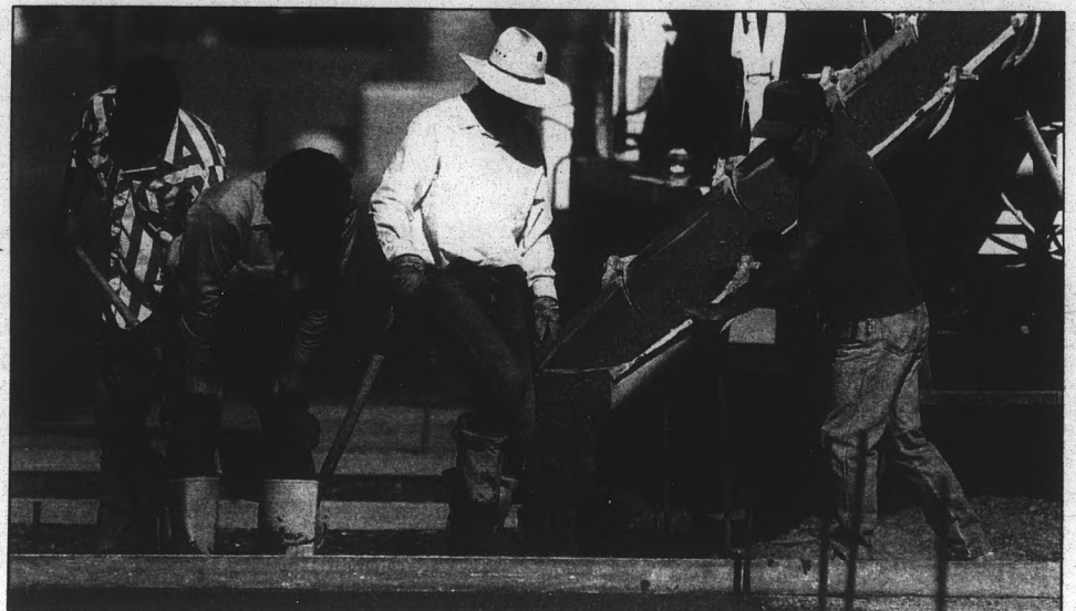
Facilities management workers pour cement during the usual round of summer construction projects on campus. This year's projects include the installation of a sprinkler system to replace the current irrigation system.
