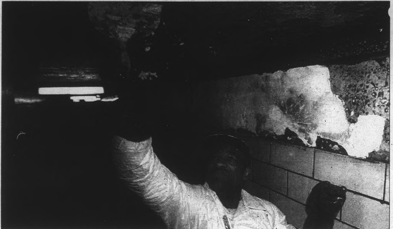
A worker scrapes burned paint off the ceiling of a Harlem apartment projects hallway Wednesday following a fire in the New York building. Associated Press
