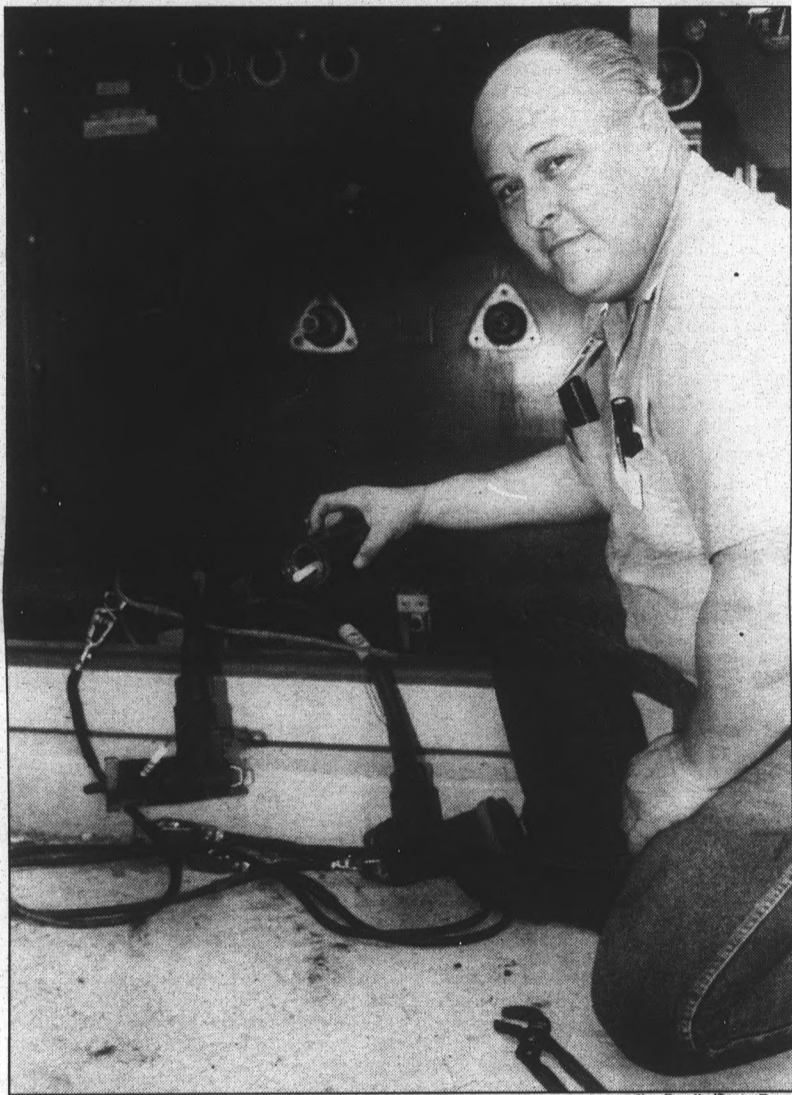
Jim Anicich, an electric shop employee with facilities management, investigates the cause of a Wednesday morning transformer blowout. Tow cables blew out in the transformer, blacking out the entire southwest quadrant of campus for more than two hours early Wednesday morning.
