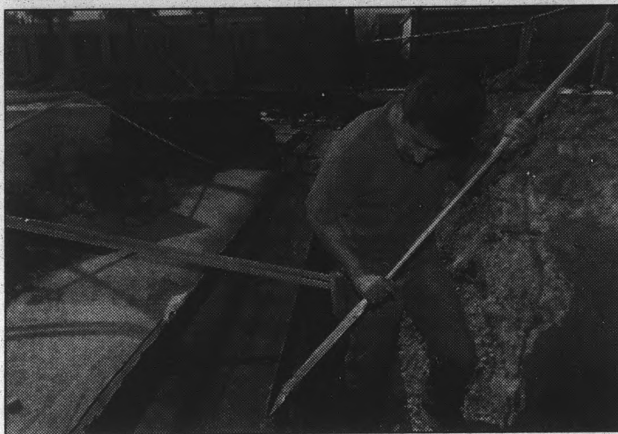
Jim Poulin/State Press A worker attempts to fix a crack between the roof and wall of the north end of the Hayden Library concourse level Tuesday afternoon. Facilities Management officials said they have found the crack, which has long been a problem for the library.
