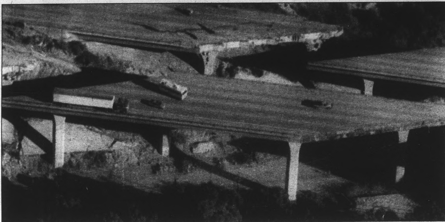
Associated Press A tractor trailer and camper are abandoned on a span of eastbound state Route 14 near Sylmar, Calif., Tuesday morning after a second portion of the interstate collapsed overnight in the wake of Monday's major earthquake that struck Southern California.
