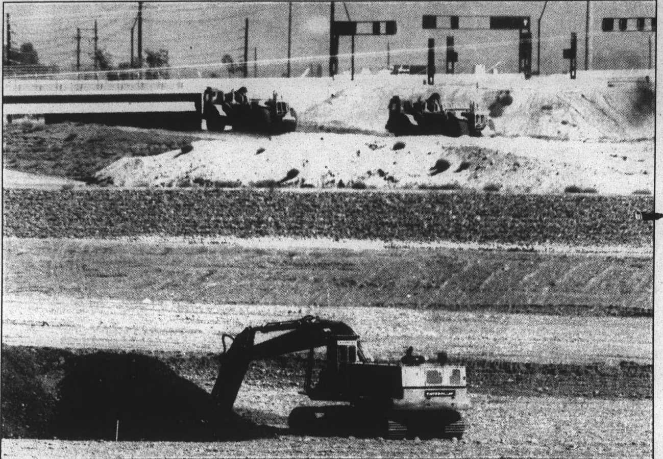
Bulldozers continue to work on clearing the path for Tempe's Rio Salado Project north of ASU. The outlook for the project appears to be better because of availability of land at no cost to the city.
