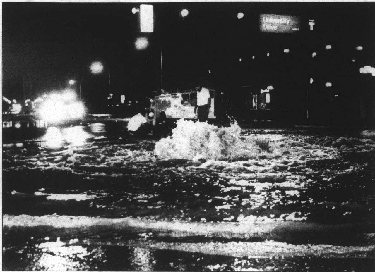
Water gushes from the ground after a water main broke at the intersection of Rural Road and University Drive Saturday night. Officials said it will be a few weeks before the intersection is back to normal after the breakage left a hole 30 feet deep and 50 feet wide.
