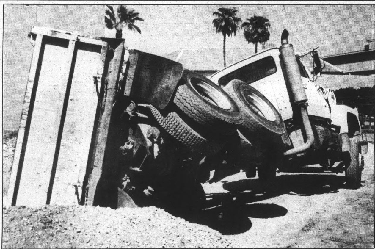
A broken hinge pin caused this truck to overturn while unloading gravel Wednesday on the site of the MU expansion project. Damage to the truck, owned by Camelback Sand and Stone, was estimated at $3,000. There were no injuries. Scott Troyanos/State Press
