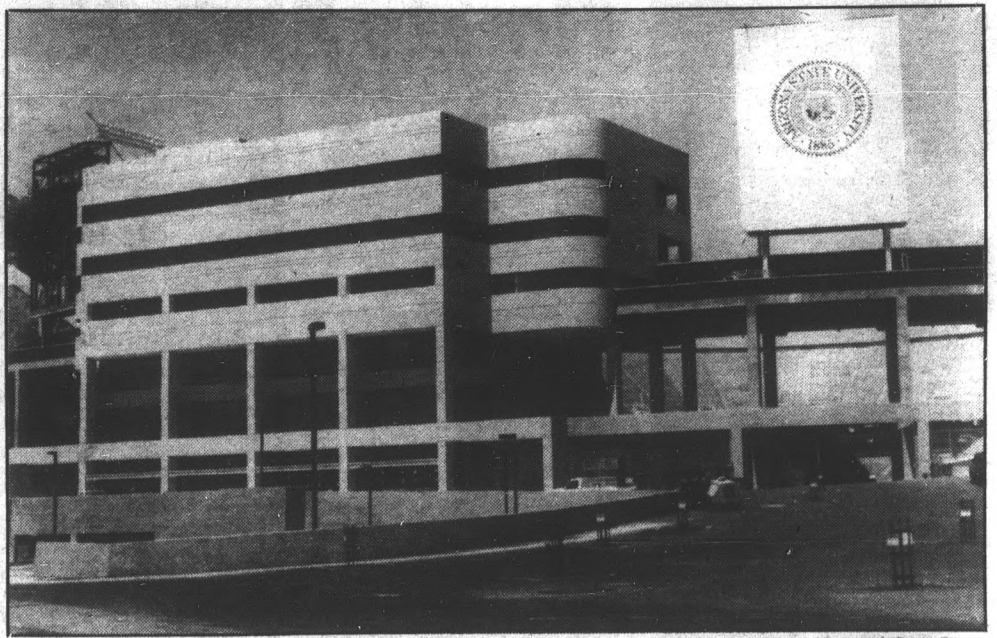
James Mumaugh/State Press Construction is nearing completion on the new Intercollegiate Athletic Complex at the south end zone of Sun Devil Stadium. Staff members will begin moving into the new structure during the first week of October.
