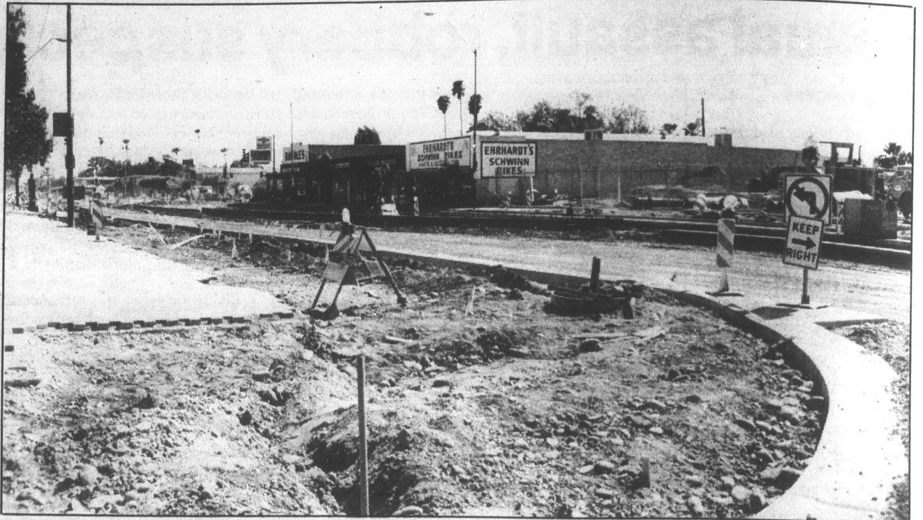
One week ago today Tempe motorists were greeted by dirt roads and construction signs at the intersections of Mill Avenue and Seventh Street. Progress has been made — most of the dirt has been removed. Sean L. Mohr/State Press
