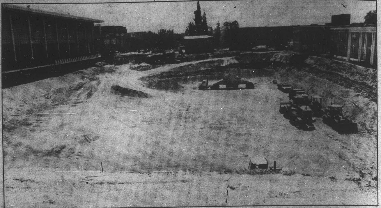
Construction crews prepare what was once West Lawn for the Hayden Library expansion.
