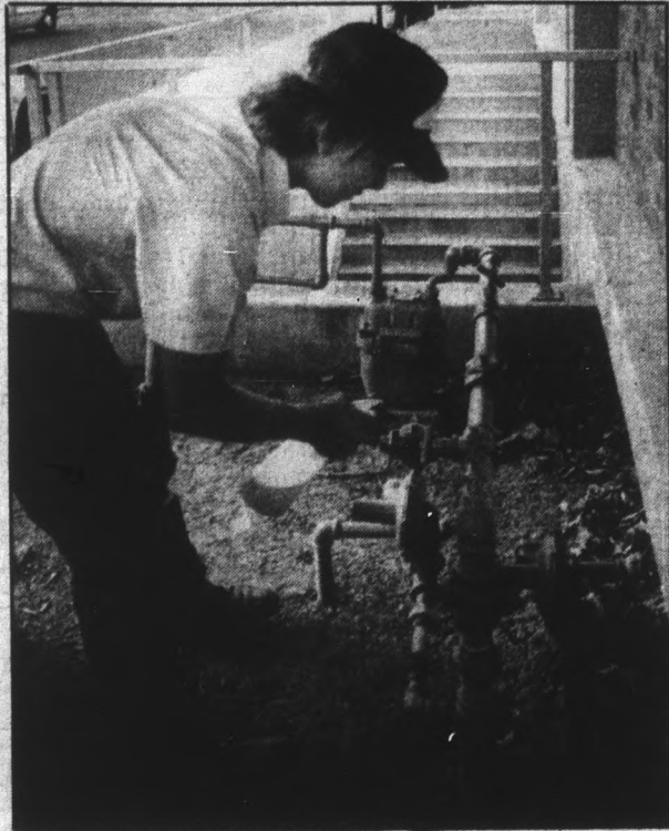
Staff photo by Kevin J. Larkin Chuck Engman of Southwest Gas Co. searches a gas line outside the Home Economics building for leaks.
