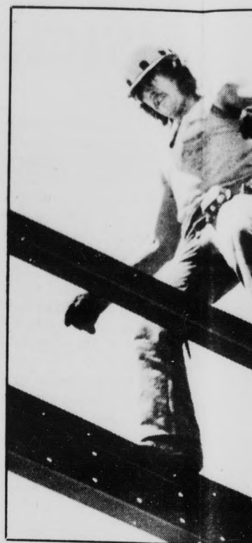
Kris Charles, a worker for Eagle Steel Erectors Inc., makes his way slowly along two steel beams.
