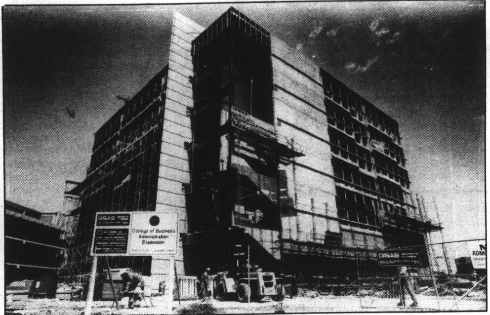
Construction of the new annex for the business college continues according to schedule. Recent rains, which flooded the basement and elevator shaft last week, have not caused any major delays.
