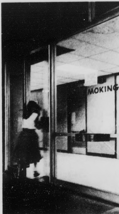
Two ASU students have been injured over the last couple years when the plate glass in the Social Science building doors have cracked due to impact with the wall.
