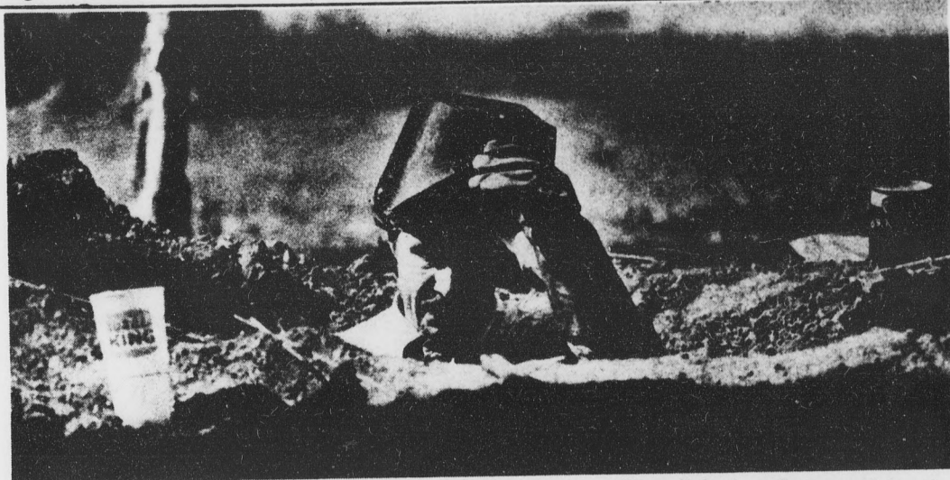
Greg Hesse, mechanics company owner, connects two gas lines 3 feet underground for the new classroom building on Terrace Road. [State Press staff photo by Sam Jones]
