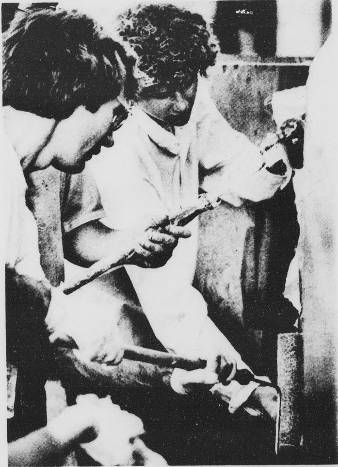
Safespace members apply one of several coats of fiberglass to the first of two wooden hulls. The vessel is being built mostly of wood to make construction easy for the amateur boat builders.
