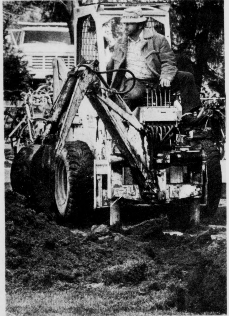
University employee Fred Zmich operates a backhoe to uncover a leaking gas line. University officials have known of the leak for over a week but have been unable to repair it because of bad weather. [State Press staff photo]
