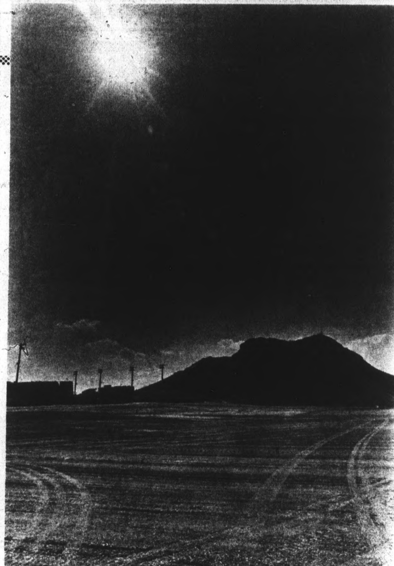
ASU is in the process of opening up several additional lots on the perimeter of the campus near Sun Devil Stadium. Officials said it took 600,000 cubic yards of dirt to construct the new lot. Photo by Craig Newman
