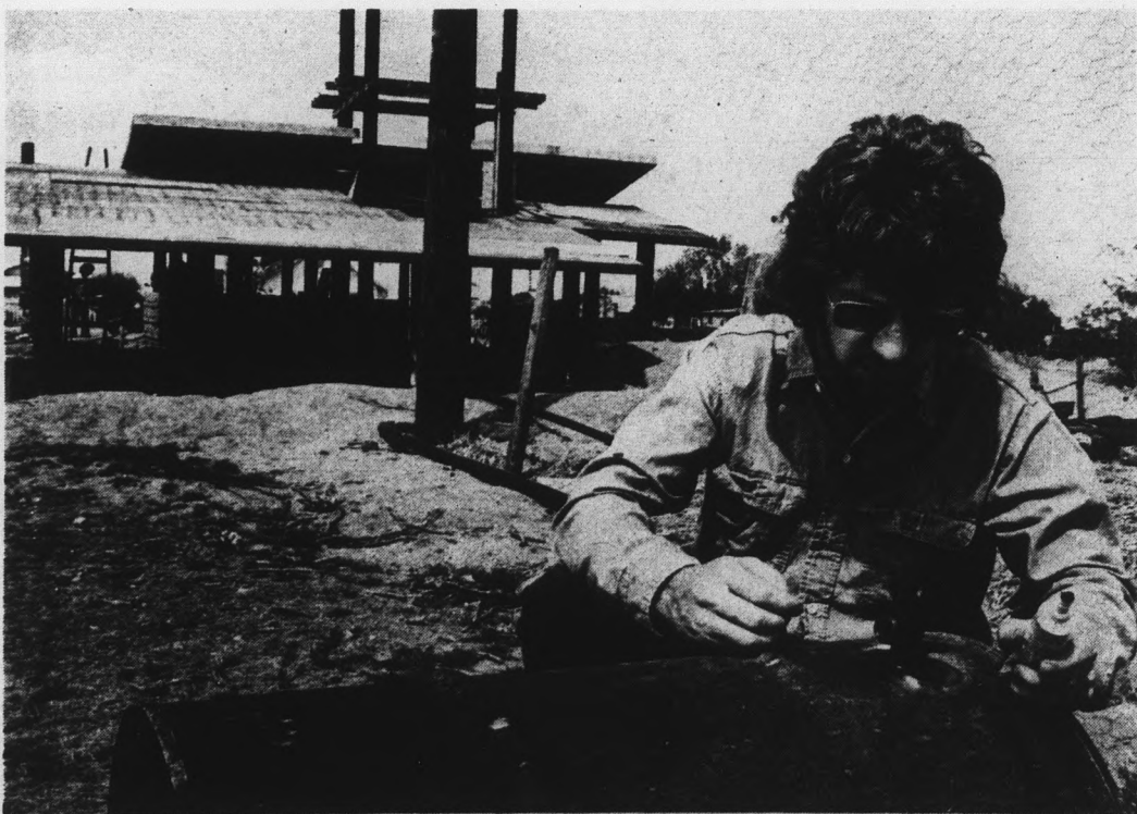
Keith Anderson, above, is constructing an experimental methane generator, which will produce cooking fuel from animal manure. The house, about 40 per cent completed, is in the background.
