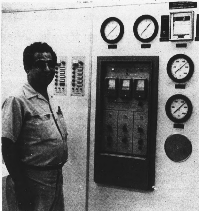
Herbert Salano, lead-shift engineer at the University's Central Plant, makes his stand in the control room. Thoughts of Freon 12, PSI and a thousand other technical goodies go through his mind . . . . .
