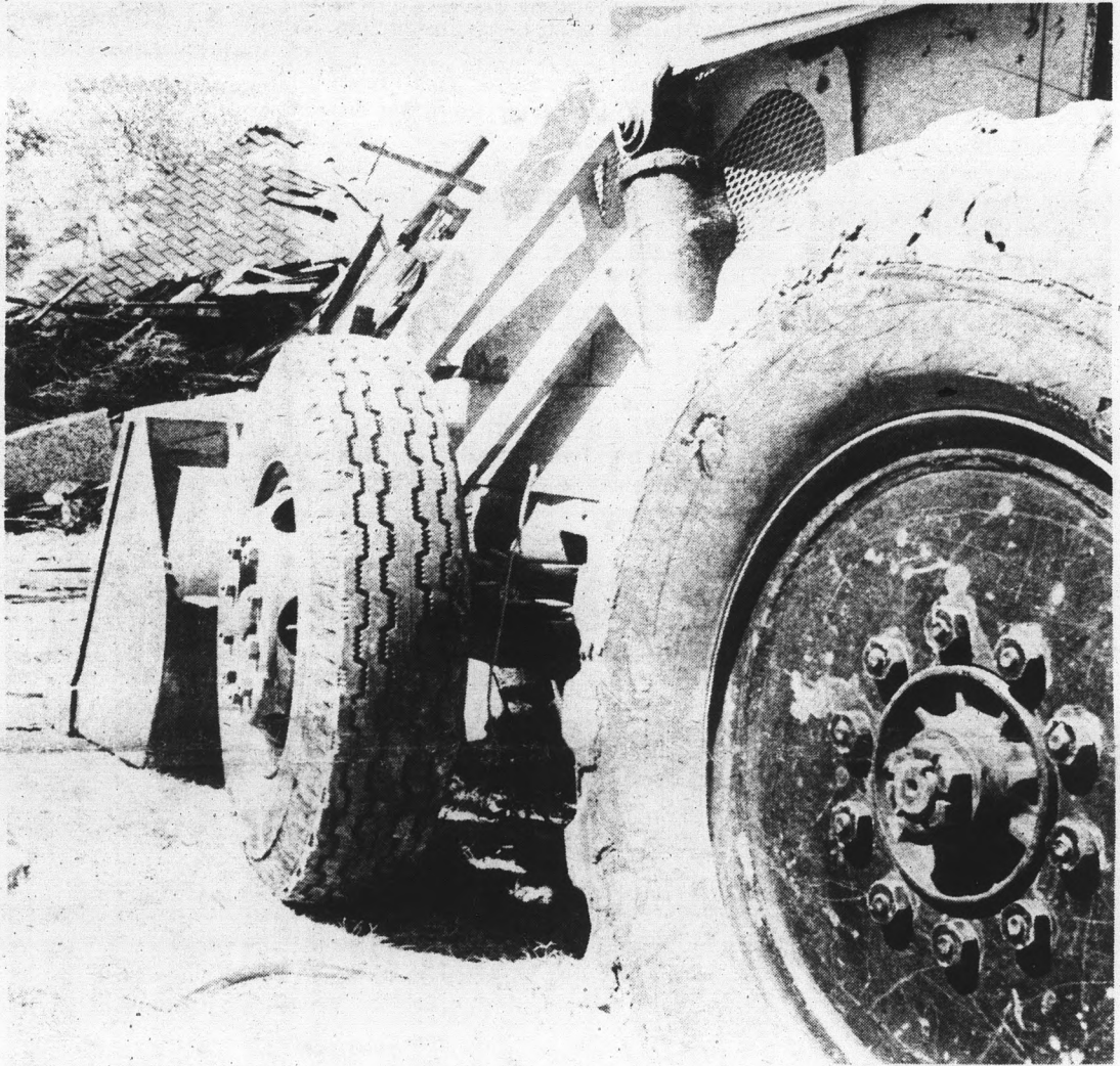
Wrecking equipment stands idle in the sun on one part of the proposed Papago Freeway route, while, at bottom left,
