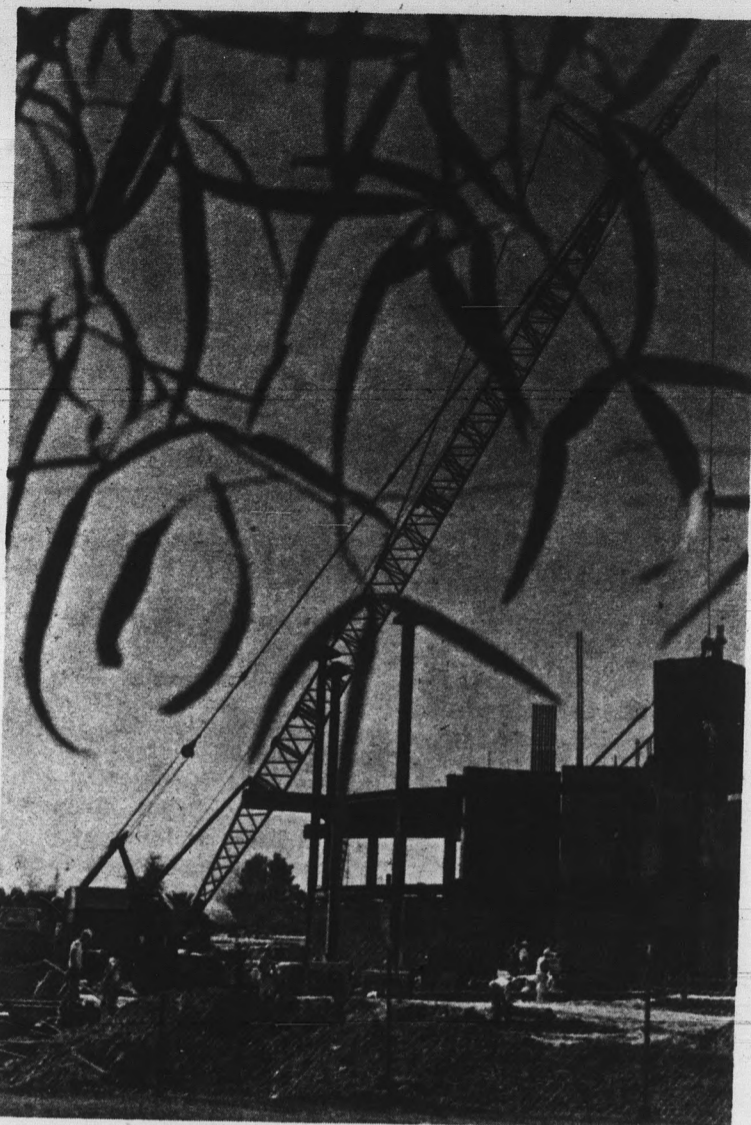
The leaves of spring frame a traditional campus sight—an extended crane—on the site of the new Music building on Mill Ave. behind Cosner Auditorium. Photo by Scott Adams
