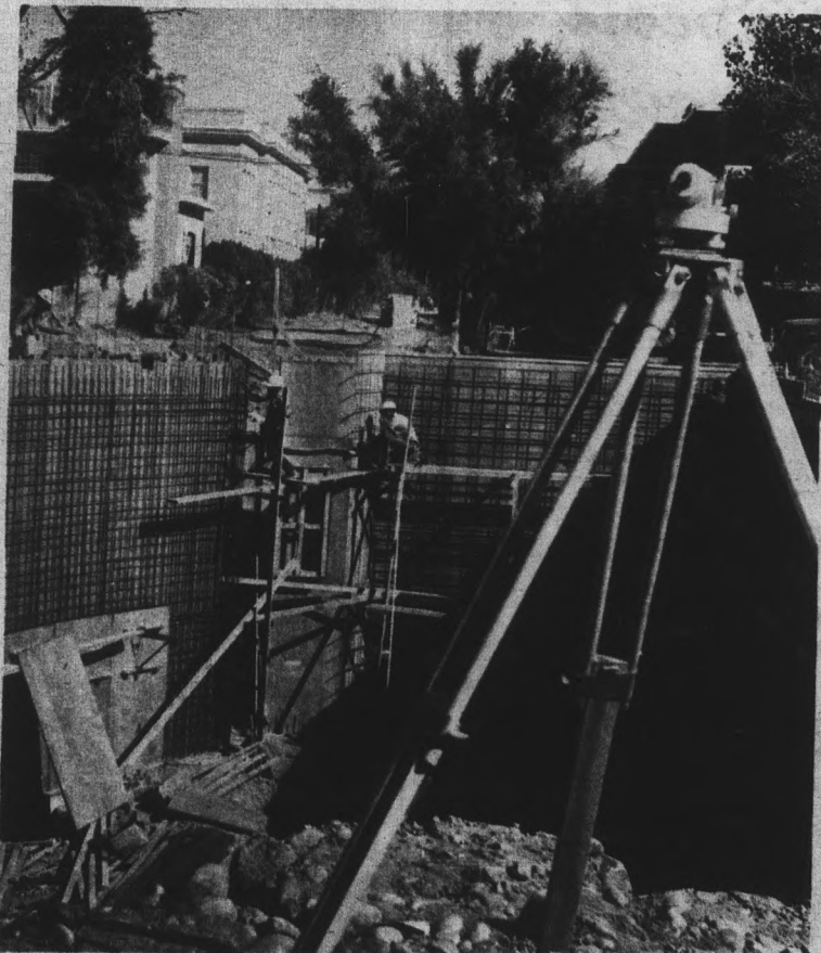
DIG IN — Construction begins on the basement level of one of the three buildings which will comprise the Art-Architecture Complex. The Complex will be located north of the new Education Building also under construction along Forest Avenue.
