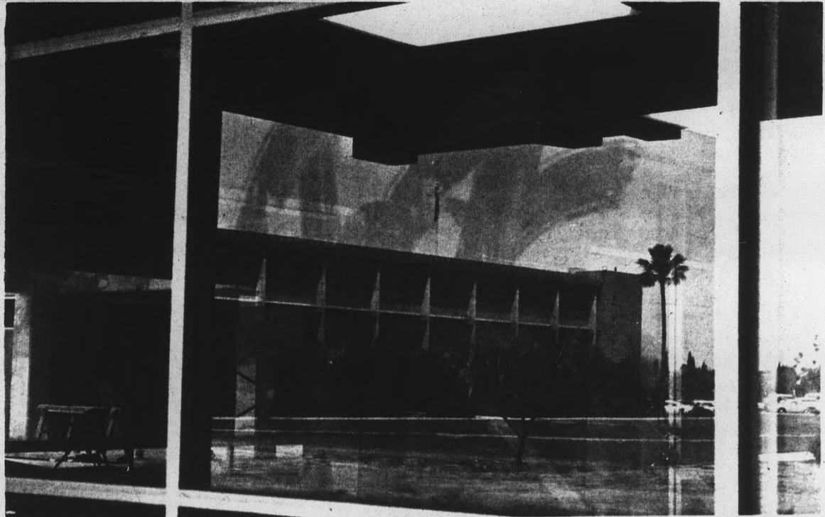
REFLECTION OF THE PAST — The familiar image of the Business Administration Building is reflected in newly-installed windows of the BA building under construction. The new structure will accommodate the college's rapidly expanding departments.
