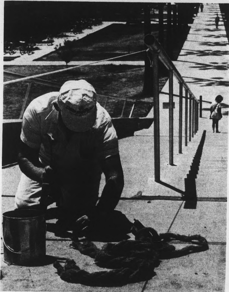
SLEAZY JOINTS — Traffic was confined to one lane on PV Bridge yesterday while workmen replaced the structure's expansion joints. The old joints were sinking below the level of the concrete.
