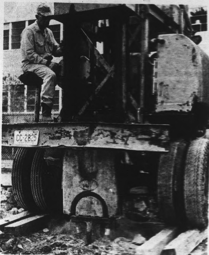
CRUNCH, CRUSH, CRASH — Machines mauled walkways in the area of Old Main yesterday as rain-dampened students scurried from class to class. The destruction is to allow new construction of utility pipes and tunnels.
