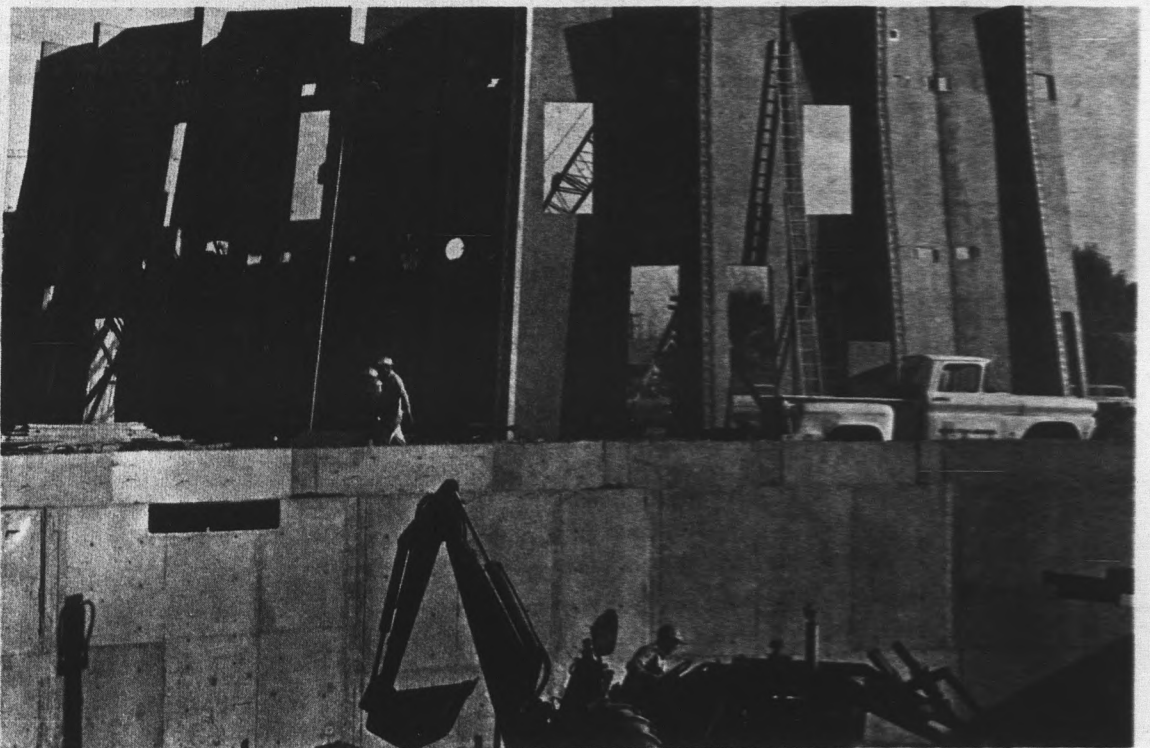
DUE PROGRESS — The underground mute court (foreground) and main center structure takes recognizable form as construction of the College of Law continues on schedule east of the campus. Single panels weigh 17 tons.
