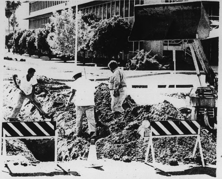
(Photo by Jack Mertes) TRAFFIC STOPPERS — Installation of a new sewer line for the women's gym has slowed traffic flow on Orange Street west of Van Ness. Since last week only one lane has been open to traffic.
