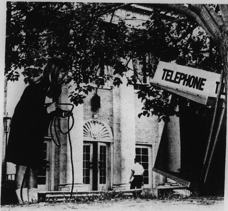
LIBRARY TELEPHONE — An outdoor phone is being installed in front of Matthews Library for students studying in the library. Until now there was no pay phone in or near the building. (Photo by John Polich)
