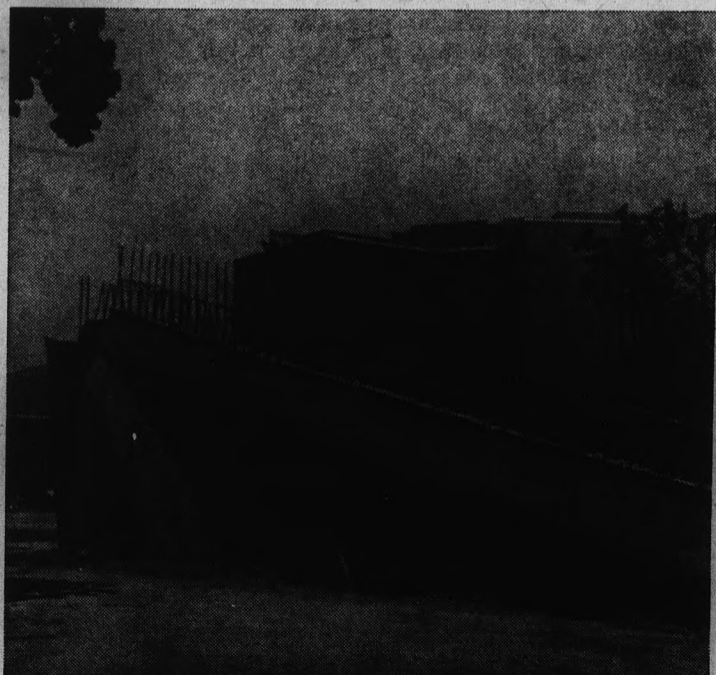
CONSTRUCTION PROGRESS —On the multi-purpose utility tunnel near 8th Street and Van Ness roles along smoothly while the new women's dorm, Palo Verde East is near completion. The proposed Palo Verde West is identical to PV East. (State Press Photo by Bill Dooley)
