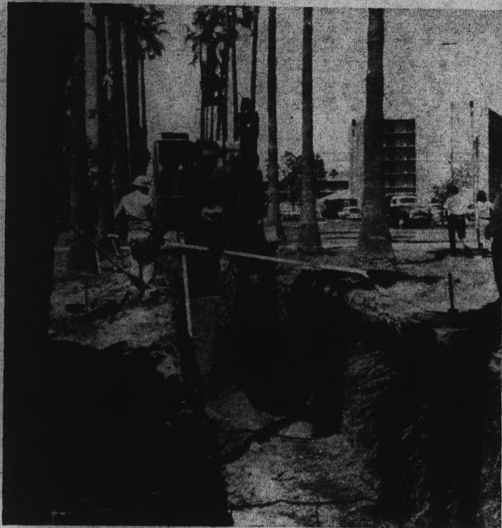
MAKE ROOM — Campus paths were cut off this week when construction crews began tunneling for utility ducts and preparing for the double-purpose overpass over Eighth street. The first campus overpass will carry heating and cooling to the Palo Verde dormitory area and aid campus pedestrians in crossing the street. ASU's tallest dormitory (right) nears exterior completion with the addition this week of seven story tall palm trees. (State Press Photo by Bill Dooley)
