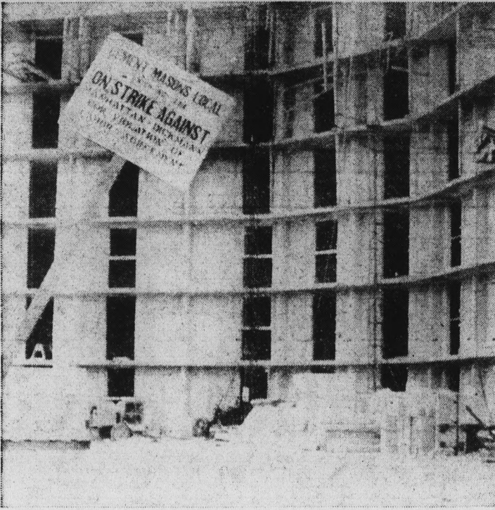
DESERTED — Work on Palo Verde East, Women's dormitory, has been stopped due to a labor dispute. Only a deserted construction site and the picket sign were on the job yesterday. (State Press Photo by Larry Ward)
