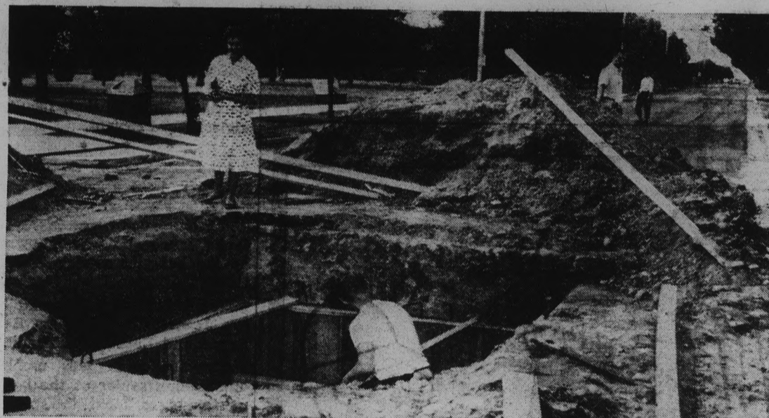
A SWITCH . . . Digging deep into College Avenue, the ASU Maintenance department is installing electrical switch equipment to establish separate power sections on campus.
