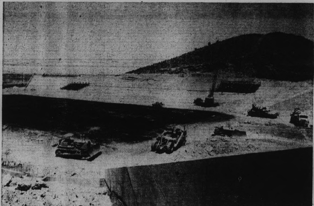
NEW HOME . . . for the Sun Devil football team, Arizona State University Stadium, shown here under construction, opened last Fall. The structure seats some 35,000 people.
