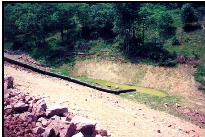
Pipe slope drain with a sediment basin at the bottom
