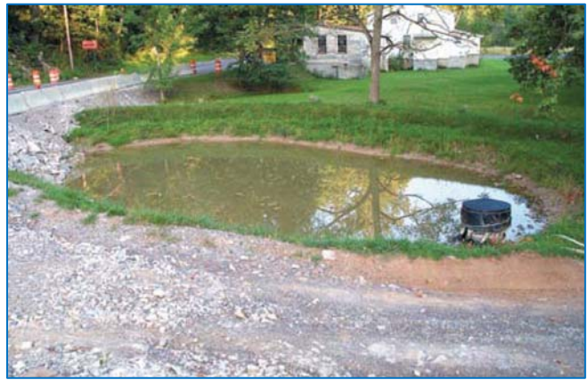
Sediment Basin. Source: Kentucky Construction Site BMP Planning and Technical Specification Manual
