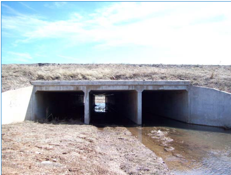
Culvert under I-17, adjacent to Tovar Trail. The left culvert could potentially be used as a pedestrian crossing to the east side of I-17.
