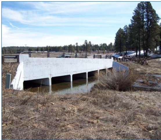
Bridge on Kachina Trail over the Pumphouse Natural Area and the Pumphouse Wash. Source: Kimley-Horn and Associates, Inc.
