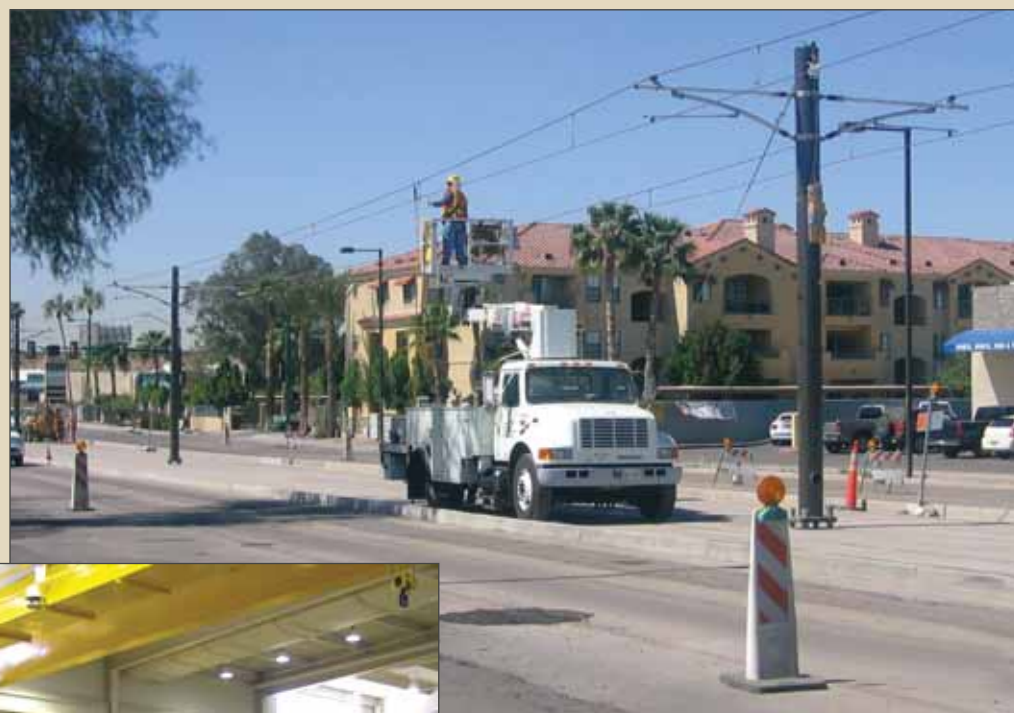
Overhead power system installed on Washington Street near 54th Street.
