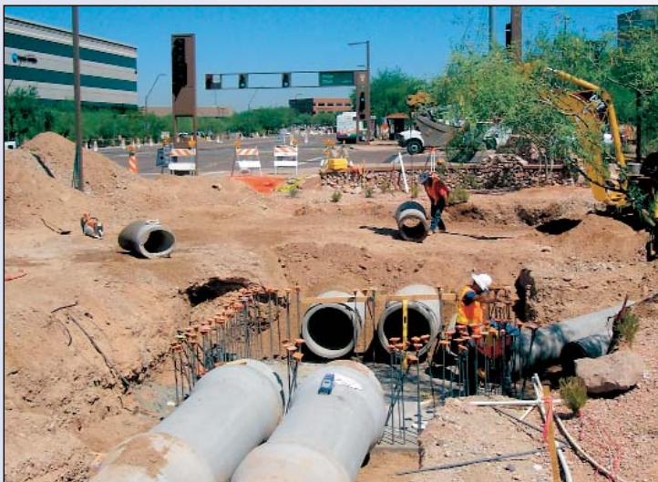
Utility relocation continues in Line Section 4 at Priest Drive and Washington Street.
