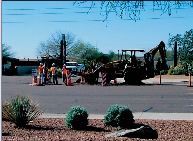
Southwest Gas works to relocate utilities in front of the Pueblo Grande Museum on Washington Street.
