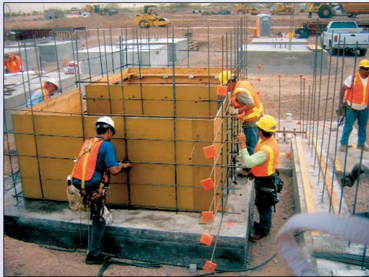
Construction continues on METRO's Maintenance and Storage Facility, located at 48th and Washington streets.
