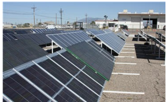
AzRISE / Tucson Electric Power (TEP) Solar Test Yard, an interdisciplinary research project to acquire and distribute data in the measurement of solar panel performance, PV production models and studies in techniques that increase the energy yield from PV systems.
