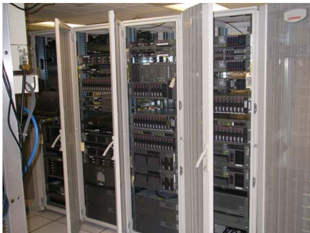
District 3 Basement Server Room
