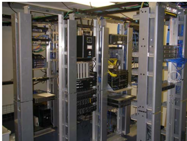
District 3 Communications Server Room
