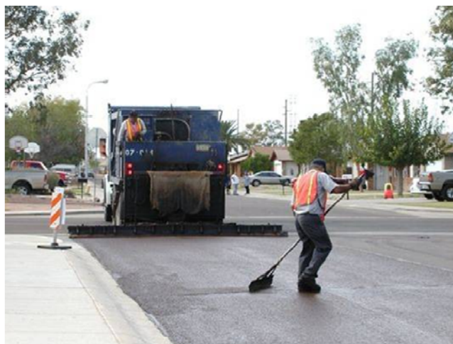
A streets crew performs maintenance work on a residential street in Peoria. The operating and maintenance costs of new infrastructure is a key factor in capital planning.
