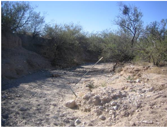
Incision and vertical banks downstream of road are significant (LM01-49-02)
