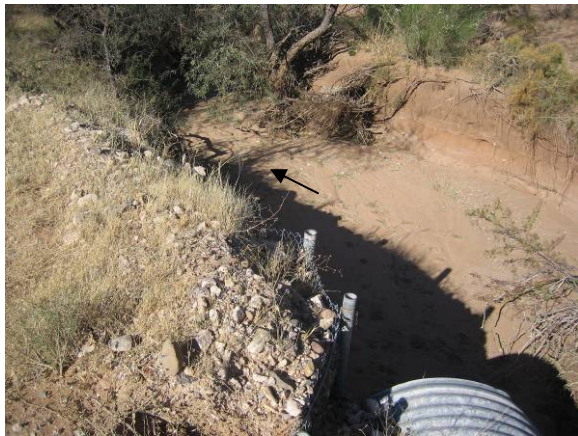
Headcut and scour hole downstream of culvert on T5 surface (LM03-23-06)
