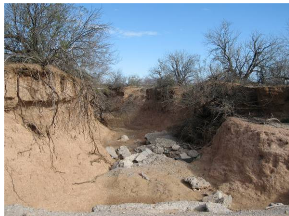
Extreme scour downstream of road, QTbf surface, facing north (LM04-12-03)
