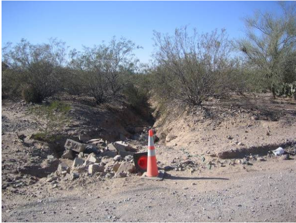
Vertical scour downstream of Salero View Road, near Three Kings Road, Qly surface (LM02-53-01)
