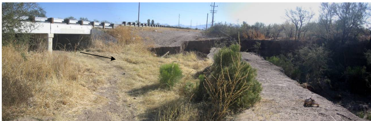
Culvert under Nogales Highway and grade control structure on unnamed wash (Pan. of LM03-68-01, 02)
