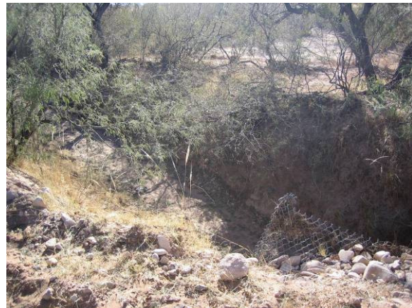
Incised wash upstream of culvert on T5 surface (LM03-23-02)
