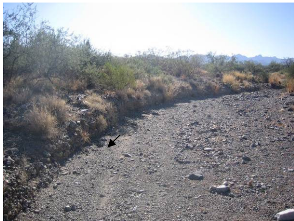
Lateral erosion along outside bend of breakout wash (LM02-16-01)
