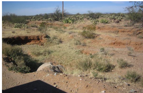
F - Headcut downstream of culvert outlet (LM03-56-01)
