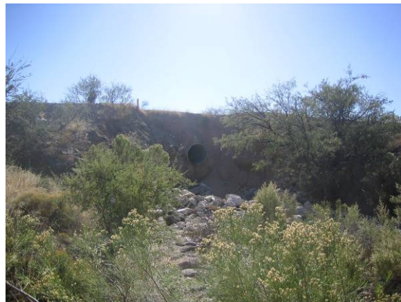
Undersized CMP east of erosion (LM02-48-01)
