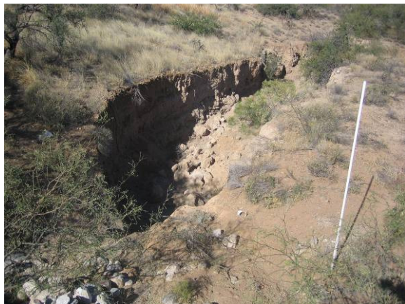
Vertical erosion downstream of Rd. (LM02-46-01)
