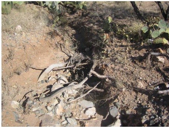
Vertical erosion on Qmo surface exposing underlying bedrock (LM02-29-02)
