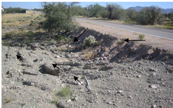
Vertical erosion developing downstream of Road on QTs surface (LM02-43-02), facing east
