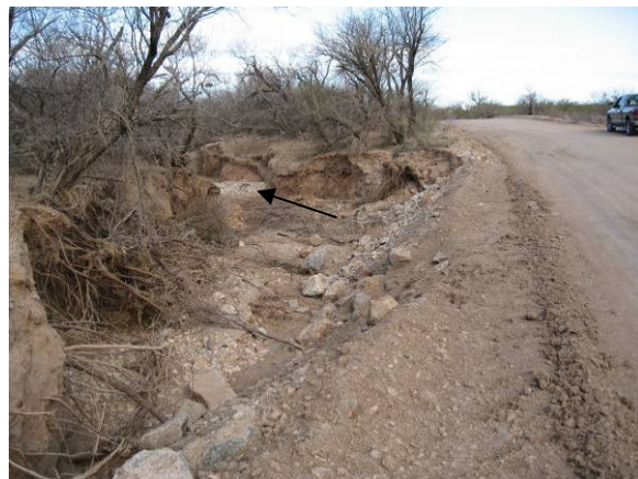
Scour downstream of Old Nogales Highway on Petty Ranch Wash, Qy Surface (LM04-02-02)
