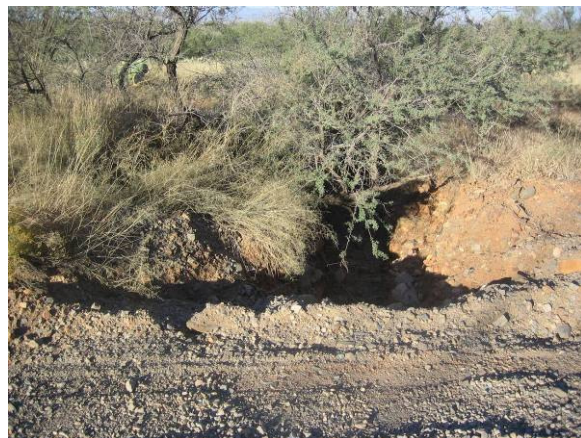
View downstream of drainage across south Houghton Road, headcutting observed below road (LM02-02-02)
