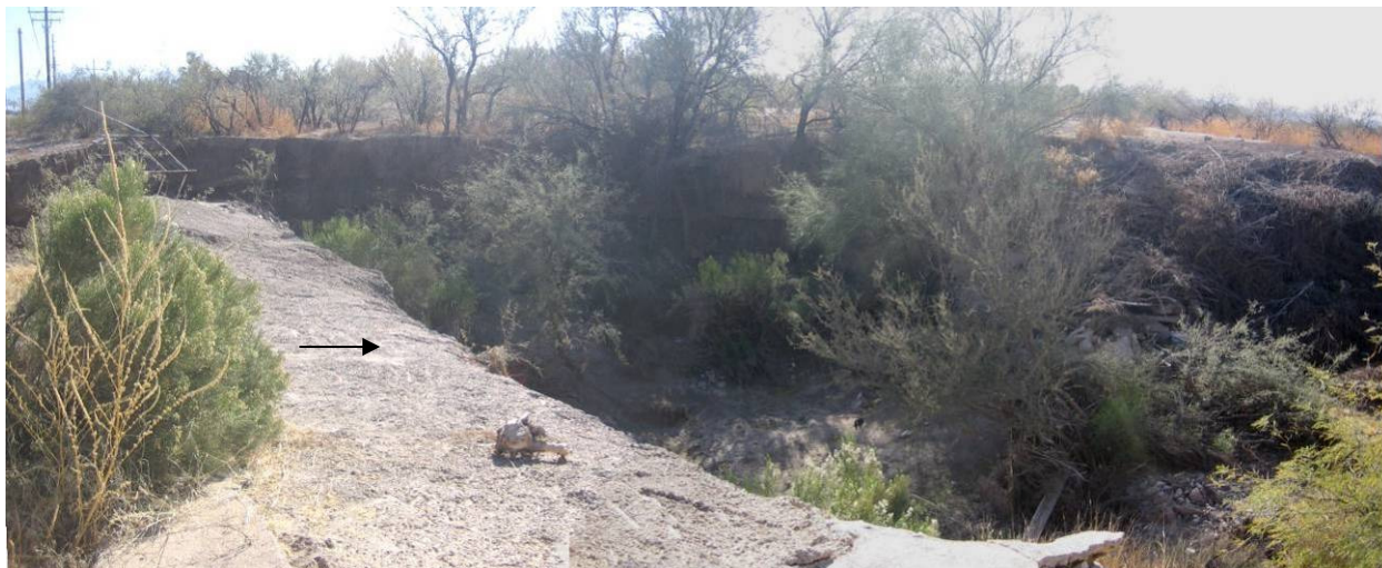
Vertical scour downstream of grade control structure on unnamed wash crossing Nogales Highway (Panorama of LM03-68-04 and 05)
