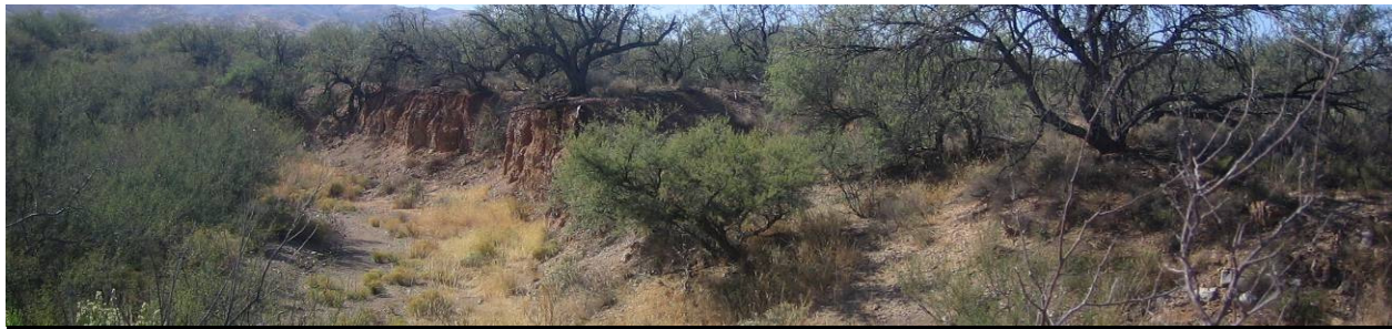
Figure 45 - Vertical banks on Qy surface upstream of Highway 83 (LM02-42-01)
