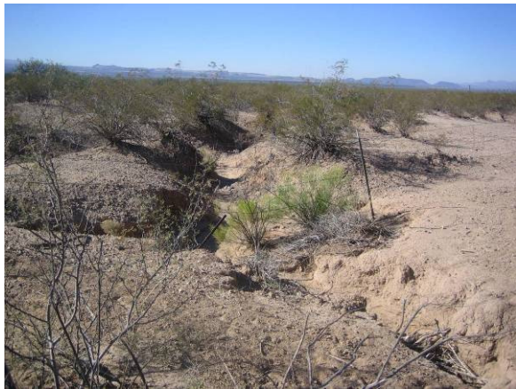
View upstream of headcutting (LM01-48-05)
