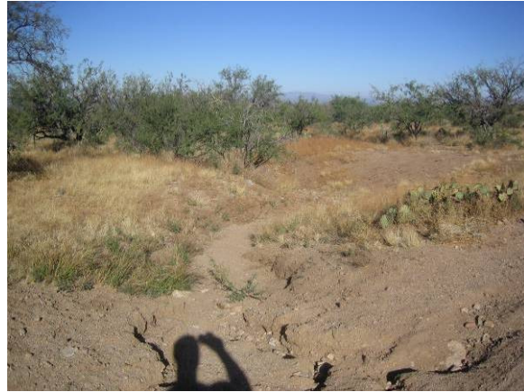
Scour formed downstream of dirt road (LM01-09-02)
