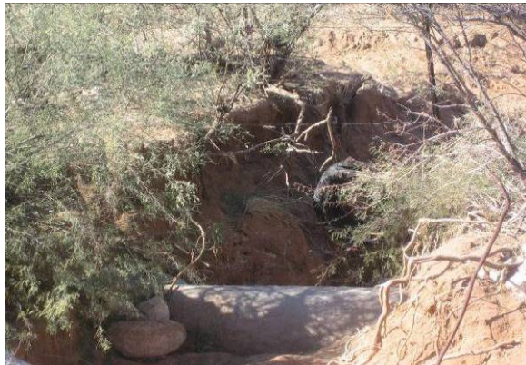
Vert. scour dstrm of rd., Qm surface (LM03-38-01)
