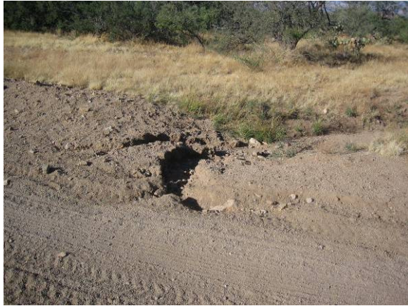
Vertical erosion at downstream edge of dirt road (LM01-09-01)
