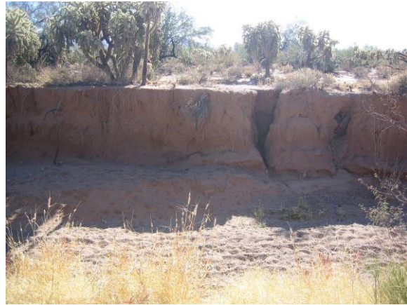
D - Vertical bank development and scouring of banks from inflow (LM03-64-01)
