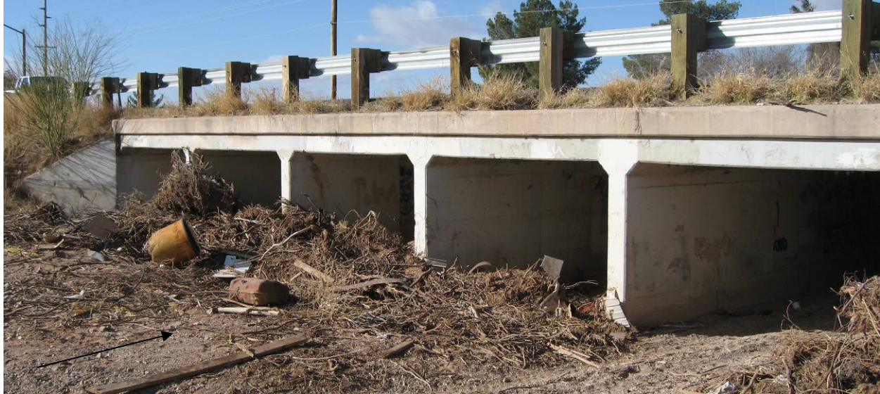
Accumulation of debris and trash upstream of Franco Wash crossing of Old Nogales Highway (LM04-07-01)
