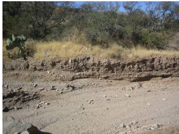
Lateral erosion (along west bank) adjacent to road on Qy surface (LM02-35-01)
