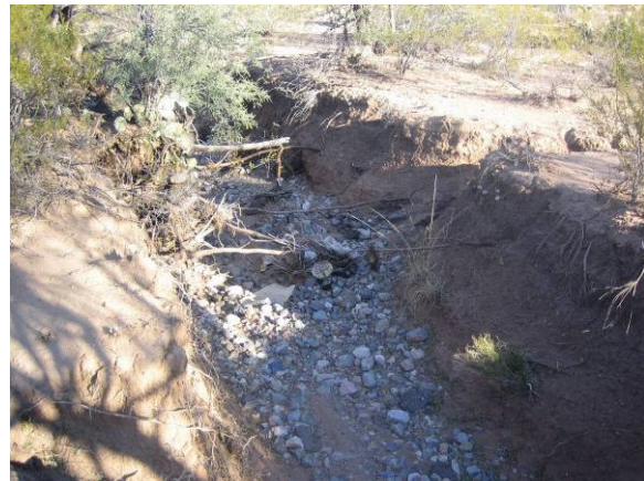
Downstream view of incising wash across Andrada Road (LM03-04-03)
