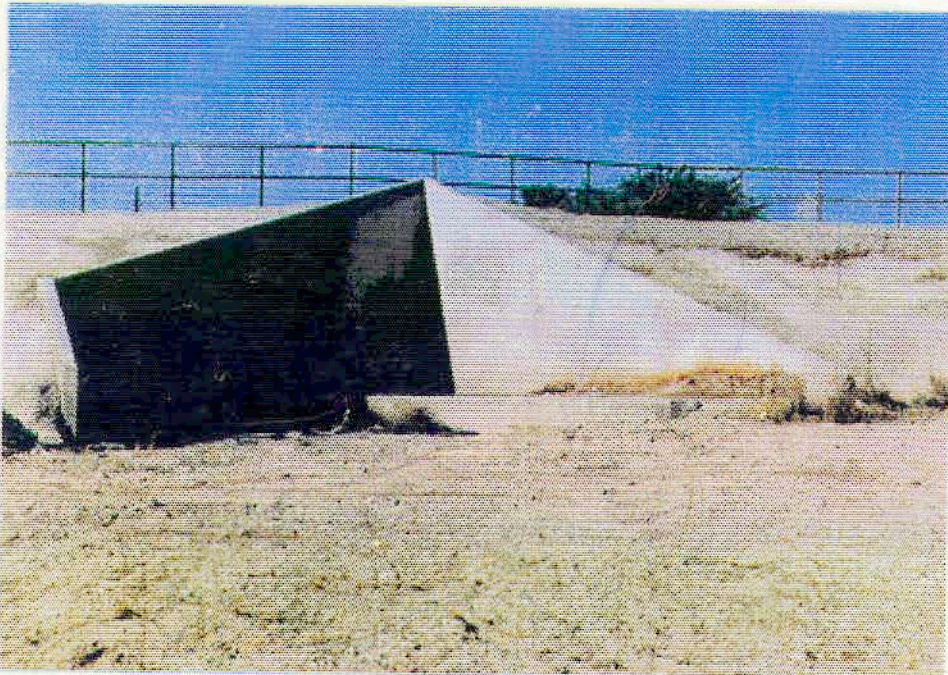
La Cholla Boulevard Storm Drain outlet at Rillito River.
