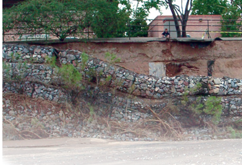
Failed bank protection. Pantano Wash, 2006.
