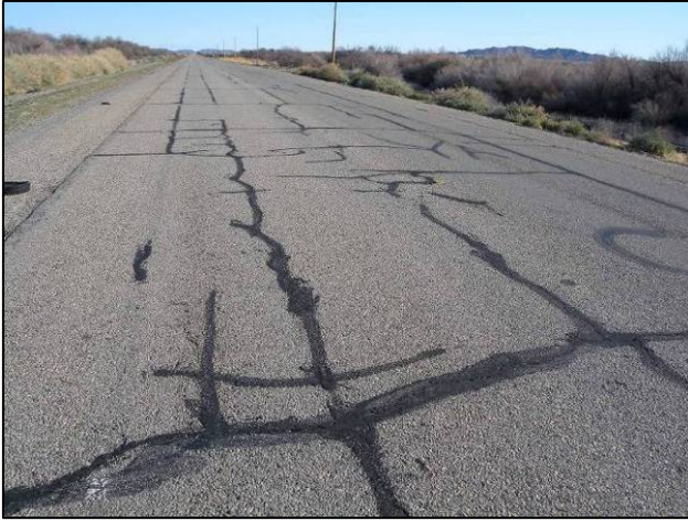
Figure 21: Mohave Road Near Milepost 1. Note Pavement Condition and Lack of Markings
