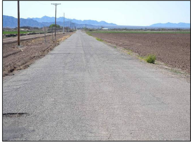
Figure 4: No Pavement Markings on Burns Road
