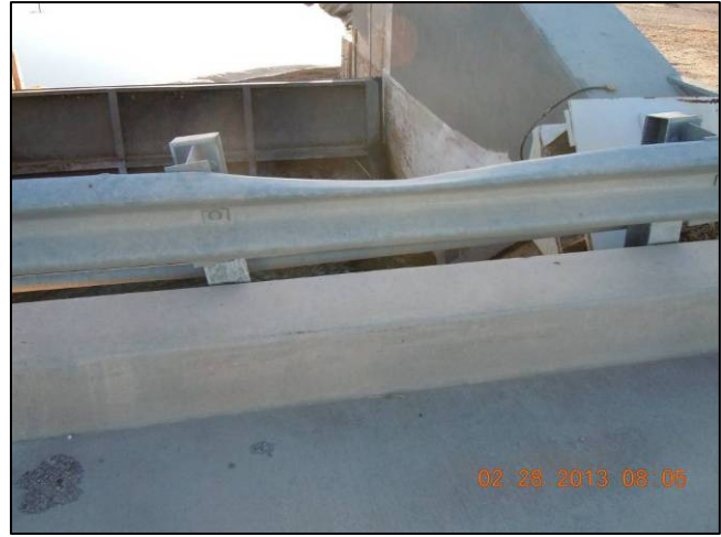
Figure 26: Damaged Guardrail at Canal Crossing near Patrick Road
