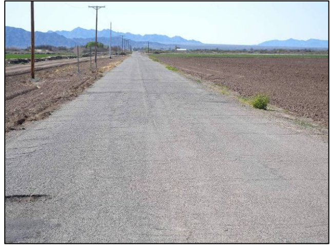
Figure 4: No Pavement Markings on Burns Road
